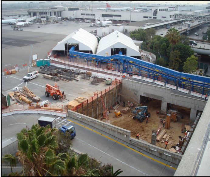
Early view of Sprung Structures at 9/27/07 opening with construction of North Matrix Building in foreground.
